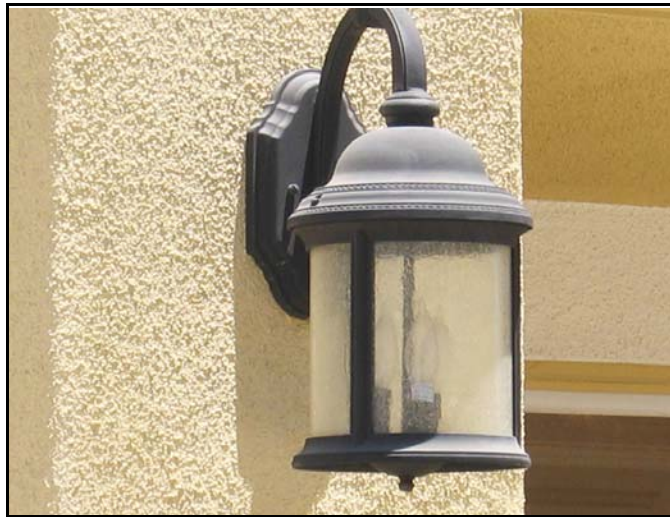
Exterior Light Fixture
