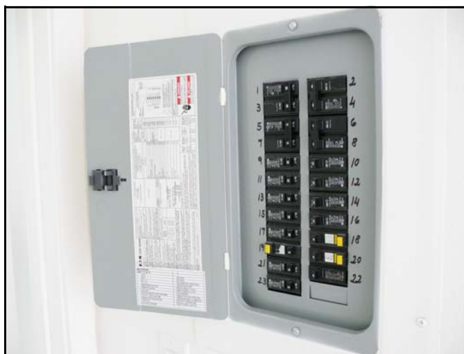
Interior Circuit Breaker Panel
