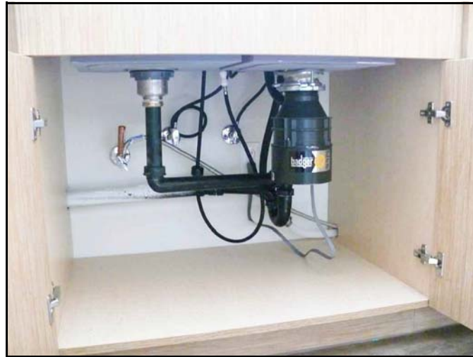
Garbage Disposal Under Kitchen Sink
