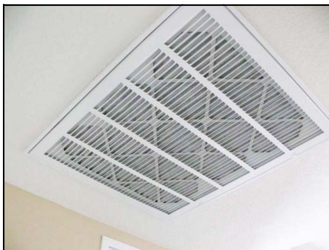
Example of an Air Filter Location
