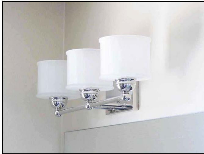
Interior Light Fixture
