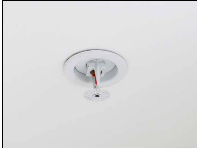
Exposed Fire Sprinkler Head
